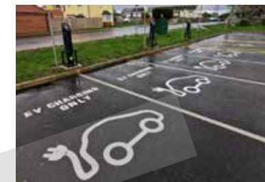
EV Chargers, Lynnsport
